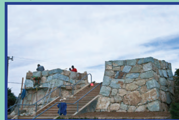
The crane lowers the final large rock in the top row/west edge of the second rampart. Note how perfectly level the cable holds the rock.
