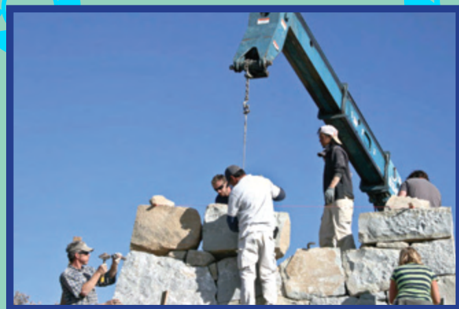
Arranging the placement of the second last rock at the front of the west rampart, Suminori Awata (dressed in white) guides the crane cable down. The rock sits firmly, with no wobble, perfectly level with the stringline at the top edge. The man in the white cap passes instructions to the crane operator.
