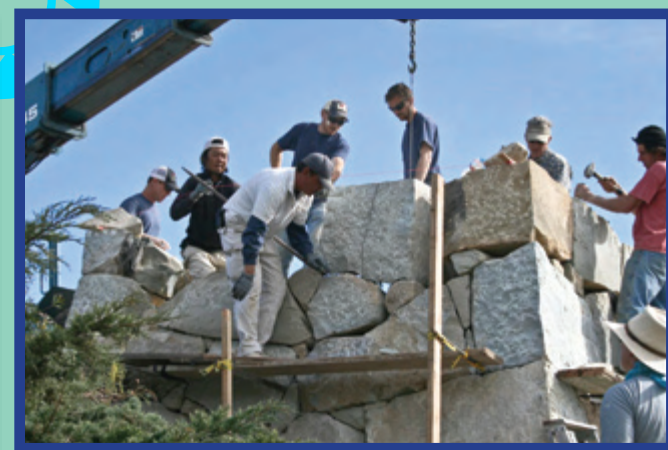
Suminori Awata's assistant shifts a boulder on the west side of the rampart with a prybar, while the crane cable holds the rock a little up. Suminori knocked one melon-sized chunk off this boulder, with one perfect sledgehammer blow. The mason at the right chisels to shape the rock placed an hour before – he was skilled enough to be able to chisel without protective eyewear.
